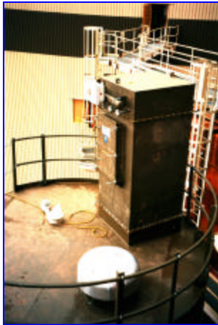
Silo Bin Vent Filter
